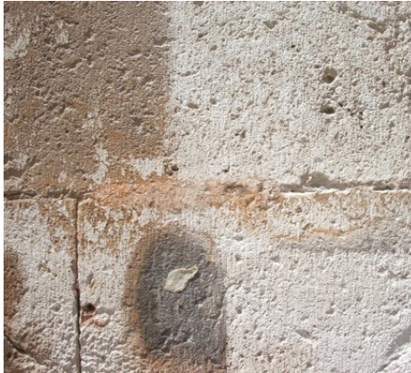
Manchas (PC4) Stains (PC4)
